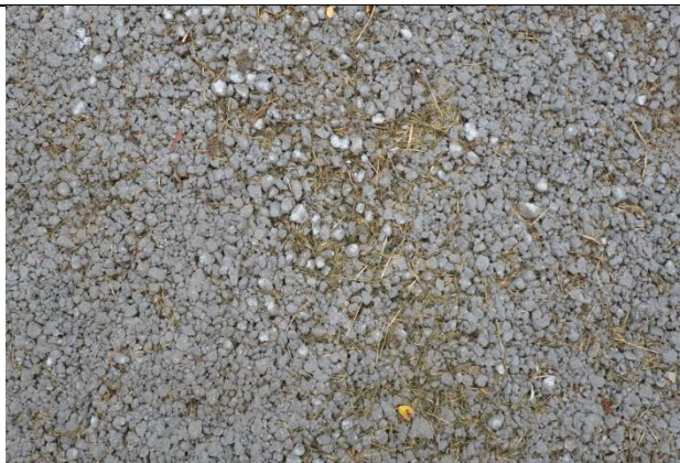
Porous concrete alongside of rain garden collects yard runoff to garden
