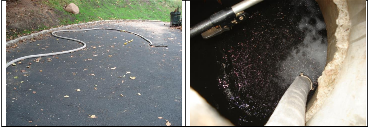
Figure 4.5. Infiltration studies for a dry well located at 383 Wyoming: filling the dry well with water from the fire hydrant and recording the fall of water level.
